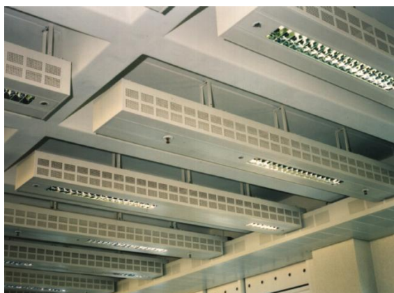
fig.3 Suspended Passive Chilled Beam
