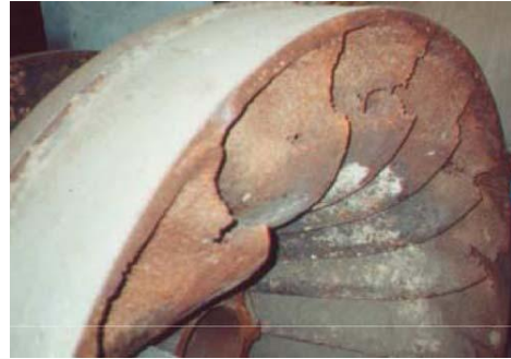
Fig. 17. Cavitation erosion of a runner
